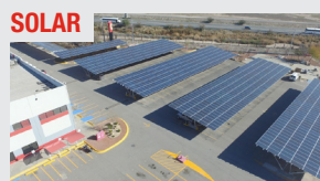
Cummins is making a significant investment in solar energy, with solar installations completed or underway at more than two dozen locations.
